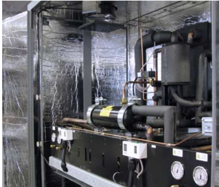
Mylar-coated sound deadening lining is standard for the larger refrigeration systems to limit noise to the room.
